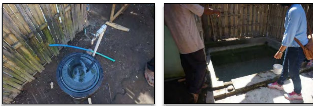
Figure 5-13 Water Reservoir And Water Hose For Connecting PDAM Water Distribution
