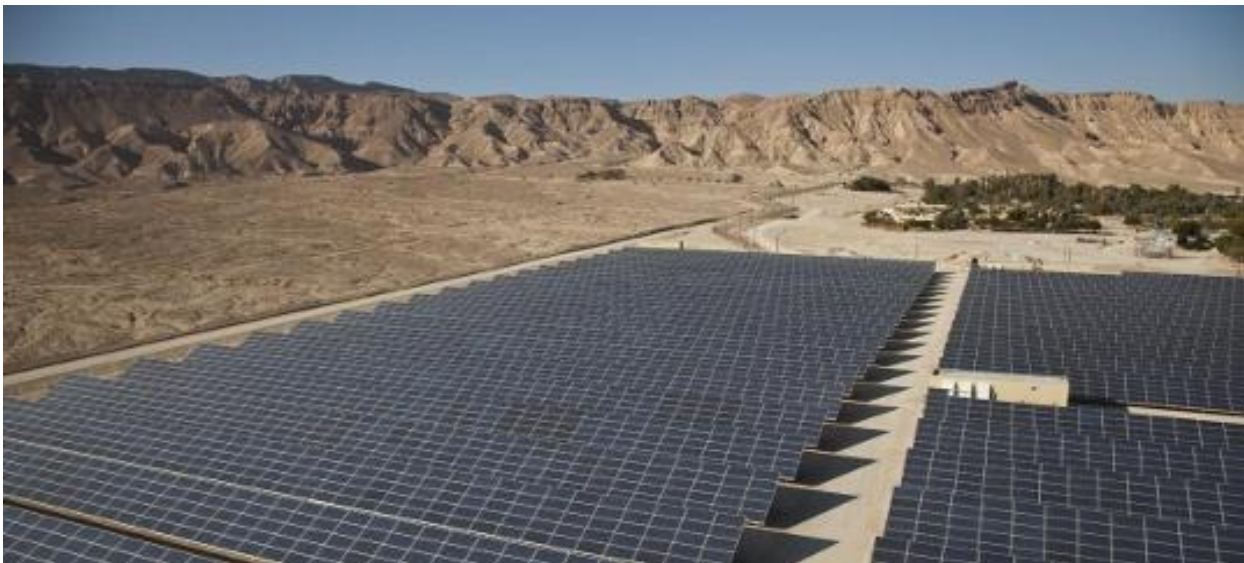
Figure 2: Typical PV Power Arrays Composed of PV Panels
