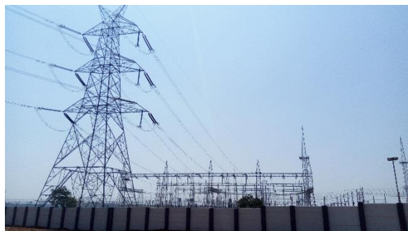
Existing Power Grid Substation at N.P. Konta
