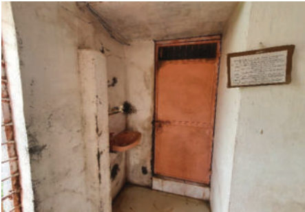
Toilet facility in Anganwadi in Jakhan village
