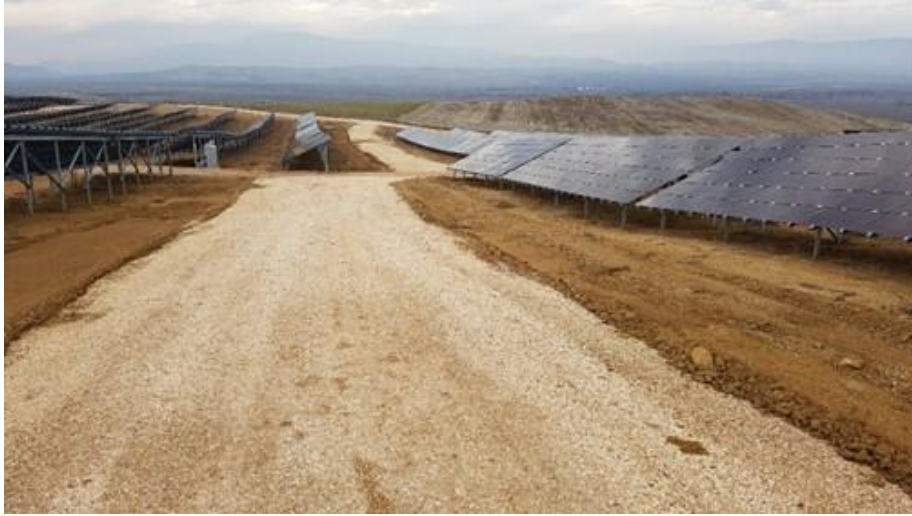
Figure 2: Photograph of Amasya Solar Power Plant
