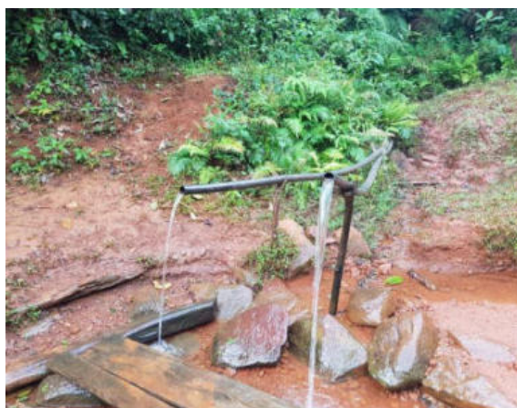
Gravity-fed water system in Xiengluang Village
