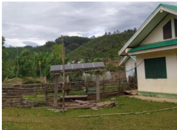
Solar cell in Dak Jom Village
