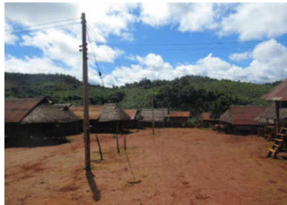
Electricity grid in Dak Yang Village
