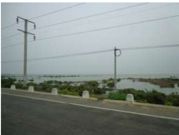
4C - The open landscape of Vankalai sanctuary bisected by causeway with visual intrusions of utility elements in vertical plane and horizontal wires/cables.
