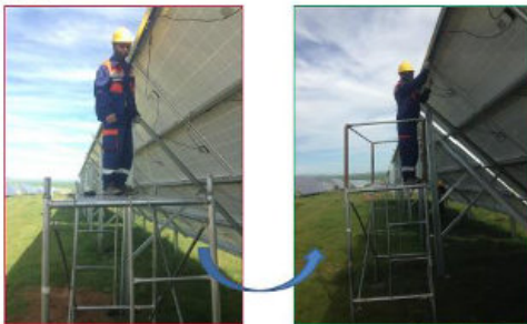
Not safe scaffold
