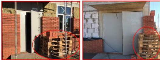
Used wrong scaffolding at masonry brick wall for Control building outside Informed to use proper scaffolds
