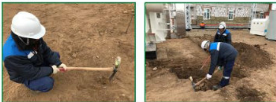
1 side cover protected of Pickaxe hand tool after continue hand digging work
