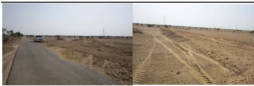
Figure 2.5 The approach road being constructed to the Project site from the Serawa - Habur road
