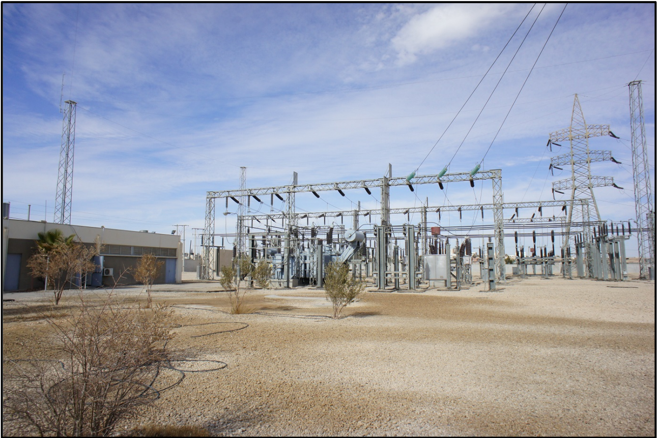
Figure 10: Typical 33/132kV Substation
