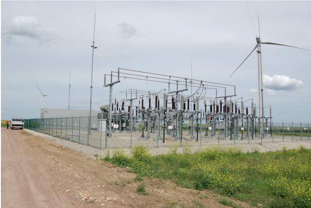
Figure 3-3: Example of Substation
