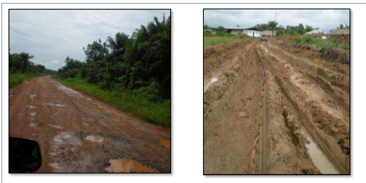
Figure 5-8: Road conditions after a period of rain.
