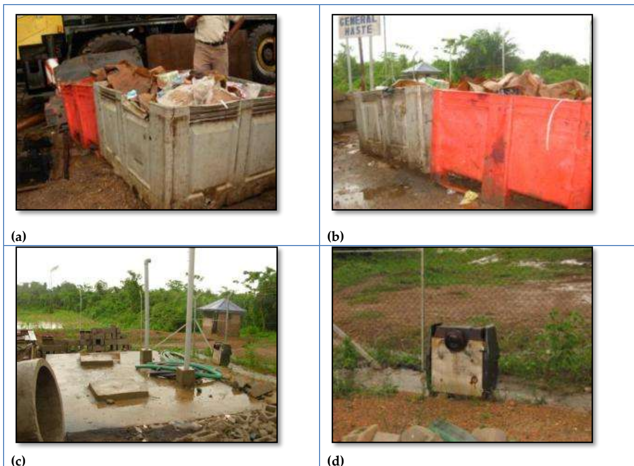
Figure 5-5: (a-b) Solid waste collection bins at main site; (c) septic tank at main site; (d) incinerator at main site that is not used anymore.
