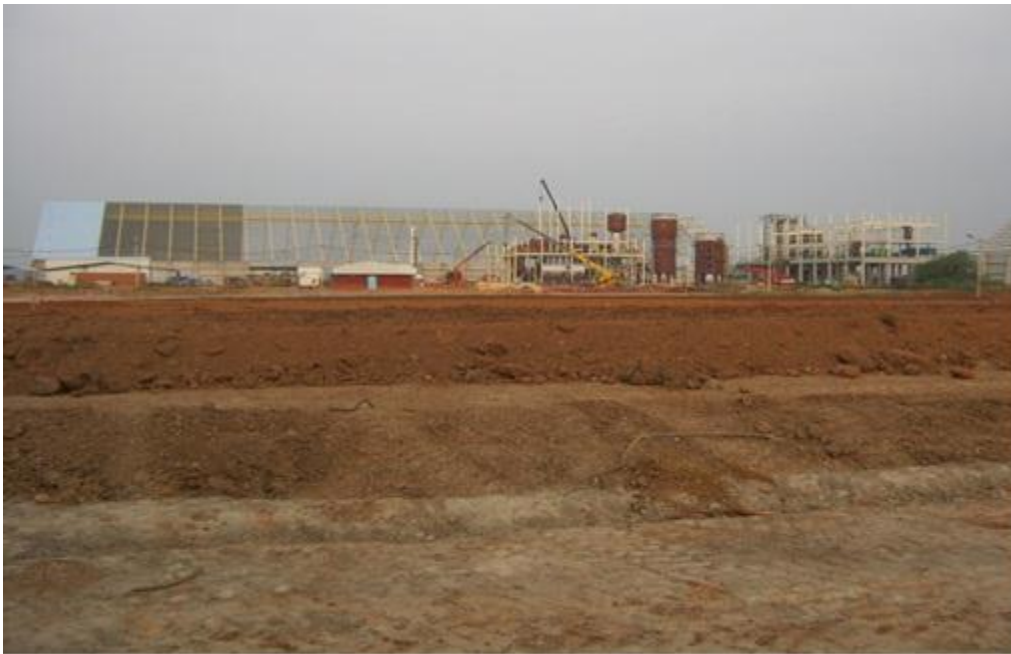
ANNEX III: View from the Paraguay River toward to crushing plant (Oct., 2012)
