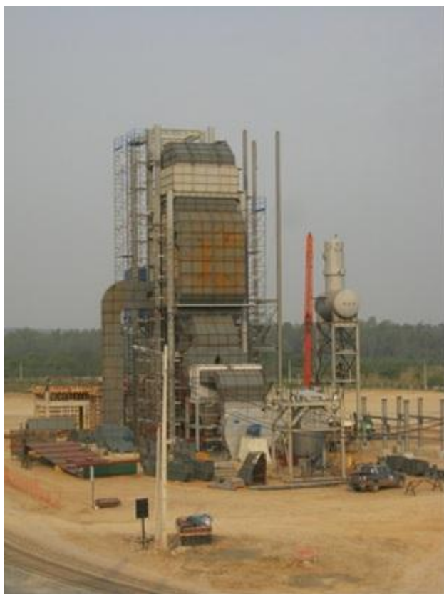
ANNEX VI: View of the biomass boiler (Oct., 2012)
