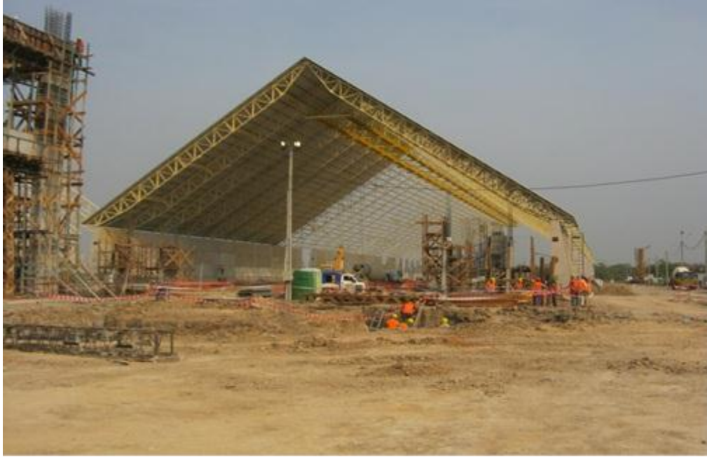
ANNEX IV: One of two raw material storage buildings under construction (Oct., 2012)
