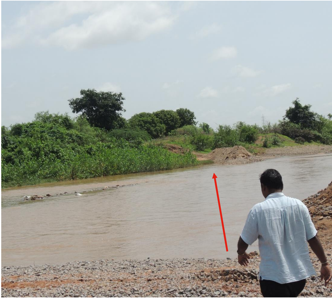
Photo 4-2 Access Road passes through Drainage
