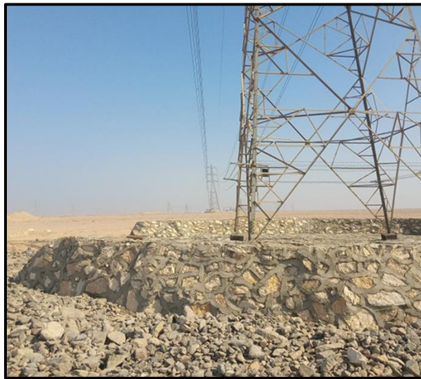
Figure 38: Base of the constructed pylons of the main OHTL in the surveyed route
