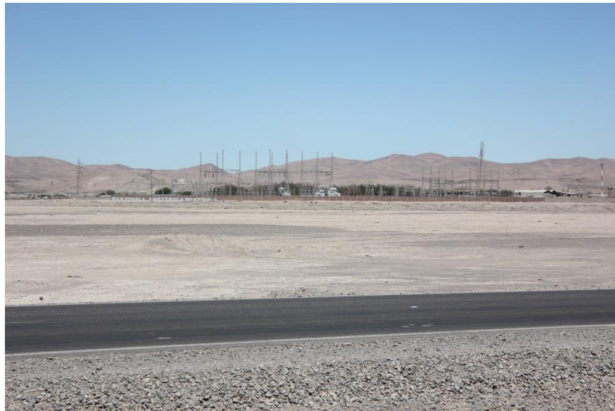
Figure 8: Existing substation both projects will connect to
