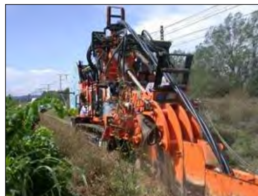
Figure 20: Sub-soil trench digging. The machine used for digging the trench to a depth of approximately 1 m
