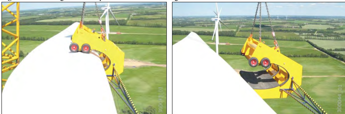
Figure 19: Holding a blade in position while it is being fastened to the hub
