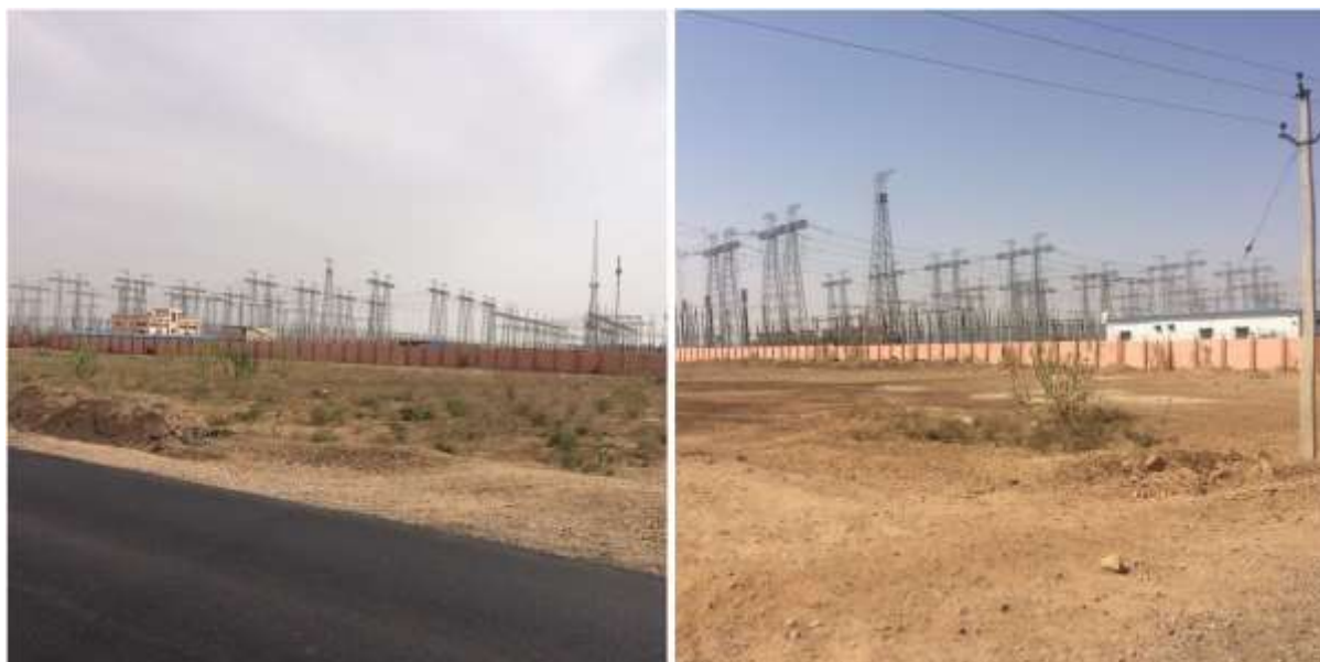
Figure 2.7 PGCIL 765 kV Grid Substation
