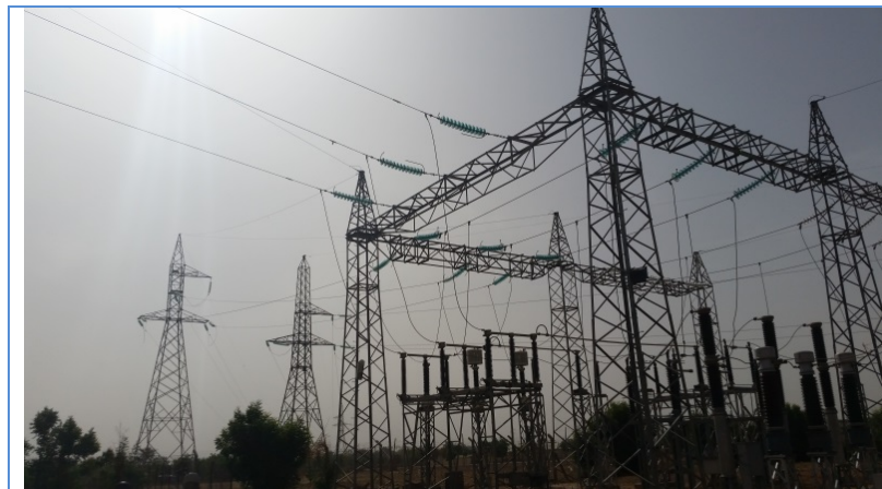
Outgoing feeder to KATSINA
