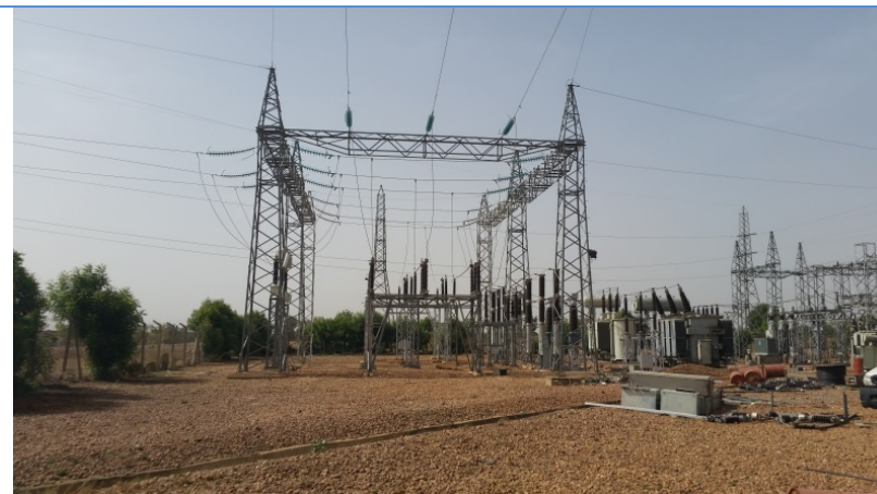
View of the whole 132 KV substation
