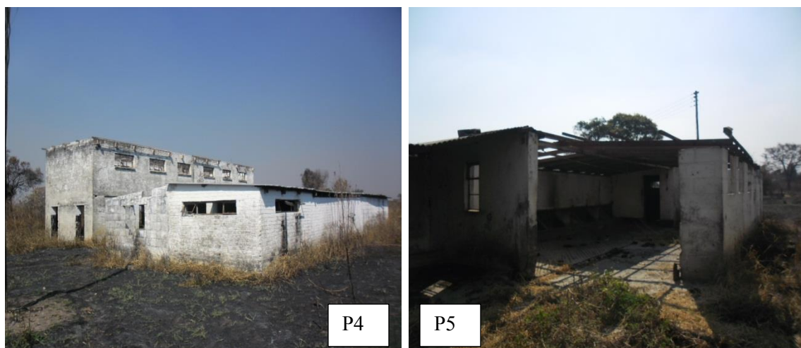
Plates 4 & 5: Showing old dilapidated infrastructure Kafubu farm.
