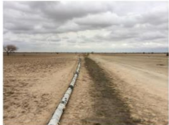
Figure 41 - - Photograph of the site in the dry season - pipe crossing the site
