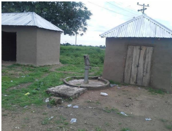
Figure 4.27: Dysfunctional borehole in Zongoro
