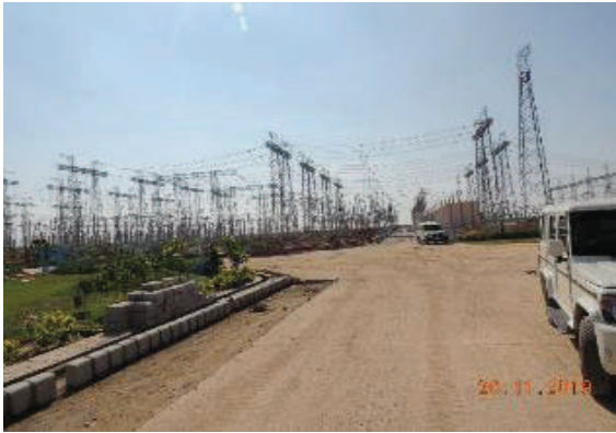
Choraniya Transmission Line
