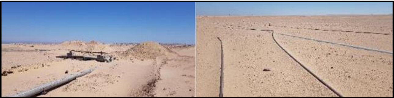
Figure 79: Petroleum Pipelines in the Project Area
