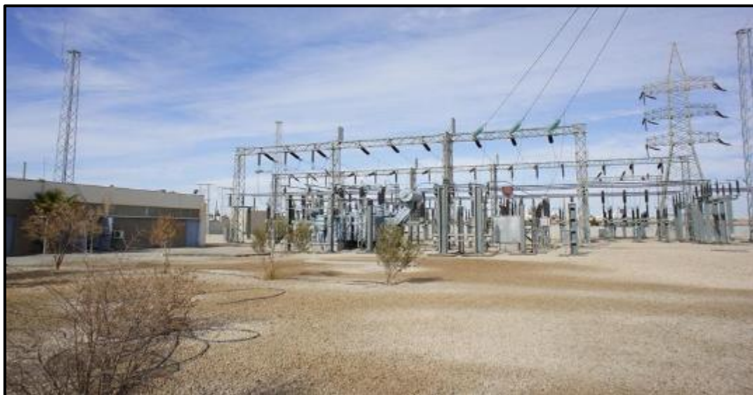
Figure 9: Typical 33/220kV Substation
