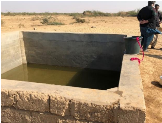
Concrete block water storage tank for livestock and domestic use.
