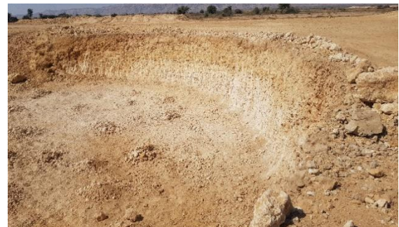
Excavation site of Gul Ahmed Wind Turbine opposite Gul Ahmed Temporary Site Facility.
