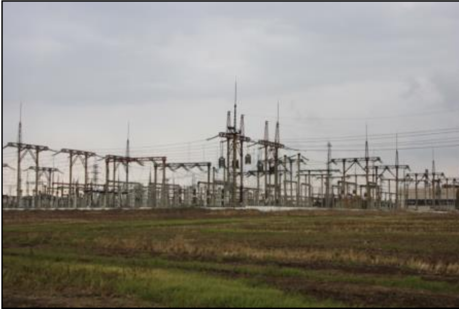
Fig. 3.26. Studies of the autumn migration of birds within the 330 kV Melitopol substation in 2016
