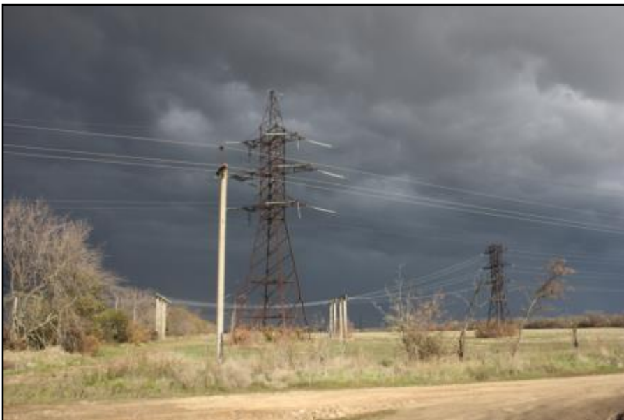
Fig. 3.27. Existing power transmission lines in the project territory
