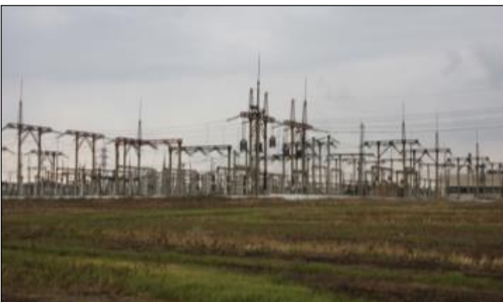
Fig.2.4. Technical landscape (Melitopol Substation)
