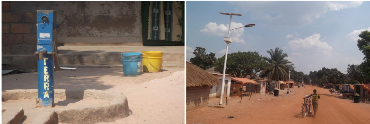
Figure 4-7: Borehole pump and Solar Lighting supplied and fitted by TERRA in Lubanda
