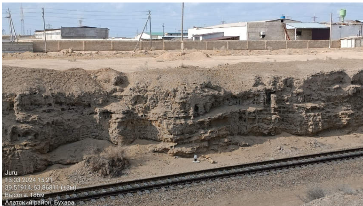
Figure 32. Loamy slope with cavities
