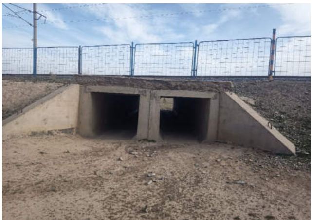
Figure 16: Double drainage under the railway
