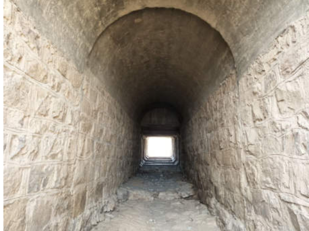
Figure 18: Most of the drainage is made up of stone masonry, 5 metres from concret
