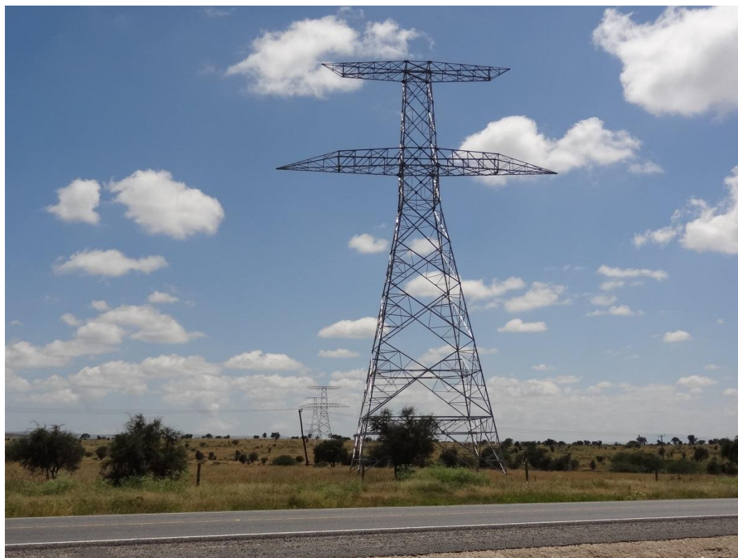
Figure 3-2: Image of a typical 220kV transmission tower
