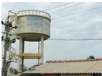
Overhead Tank at Veligallu village
