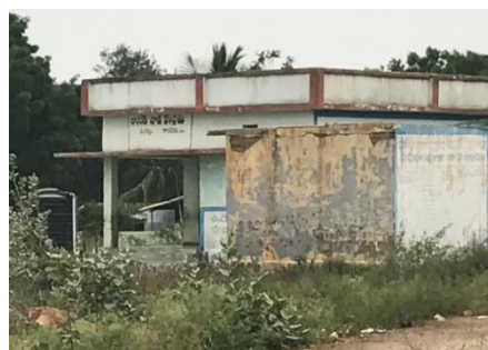
RO Water Filter reservoir at Veligallu
